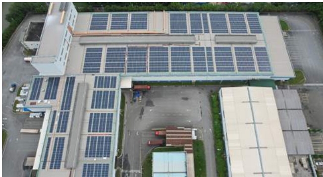
Two major projects to install around 8,000 solar panels were completed at sites in China – helping to accelerate our ambition of cutting carbon emissions in half by 2030. The panels were installed at two of our Decorative Paints plants – more than 5,000 in Shanghai and almost 3,000 in Guangzhou – representing further progress for our greener manufacturing plans.
