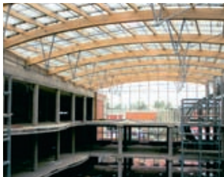
Fig. 3 Roof framing for atrium from lam beams for a trade and exhibition centre in Lahta, span up to 24 m.
