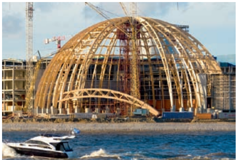
Fig.2. Timber structures, meridional ribs with chord 60 m for the water park dome section (dome diameter 90 m) in St. Petersburg's 300-Year Anniversary Park.
