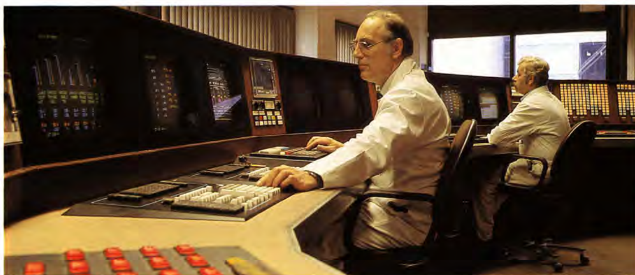
Nerve center of our new membrane electrolysis plant at Rotterdam. The staff manning this control room monitor the production process and are ready to take remedial action in a variety of situations, including such as endanger environment and safety.
