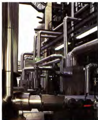
Detail view of the maze of pipes in Bergen, Belgium, fatty amines plant.
