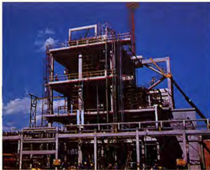
Akzo's Crystex® insoluble sulfur capacity is undergoing expansion, with a new manufacturing facility under construction in Brazil.
