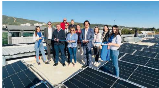
More than 2,300 solar panels have been installed at our Izmir powder coatings factory in Türkiye. The factory roof has been covered with 5,250 square meters of solar panels, contributing to our ambition of using 100% renewable electricity by 2030. We were proud to become the first company to invest in solar energy in the Aegean Free Trade Zone.
